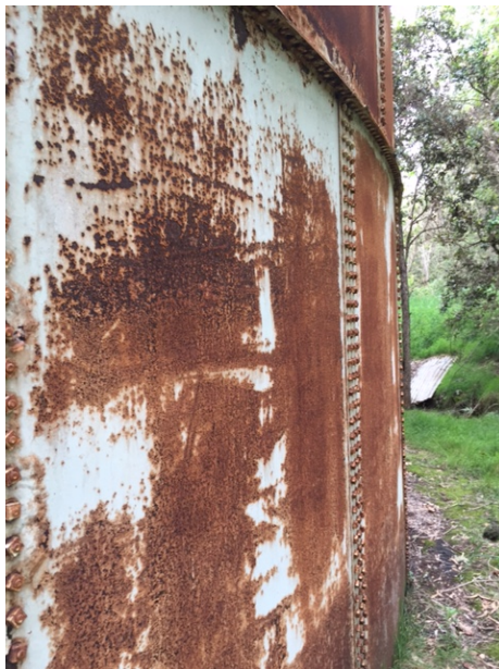
Photo 2. LCP grey paint in poor condition on the lower water tank.
