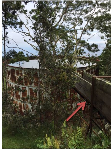
Photo 1. ACM grey sealant on large gutter underside of upper tank.
