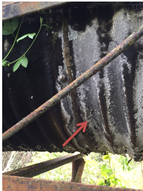
Photo 2. Close-up of grey sealant on large gutter underside of lower tank.
