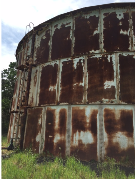
Photo 1. LCP grey paint in poor condition on the upper water tank.
